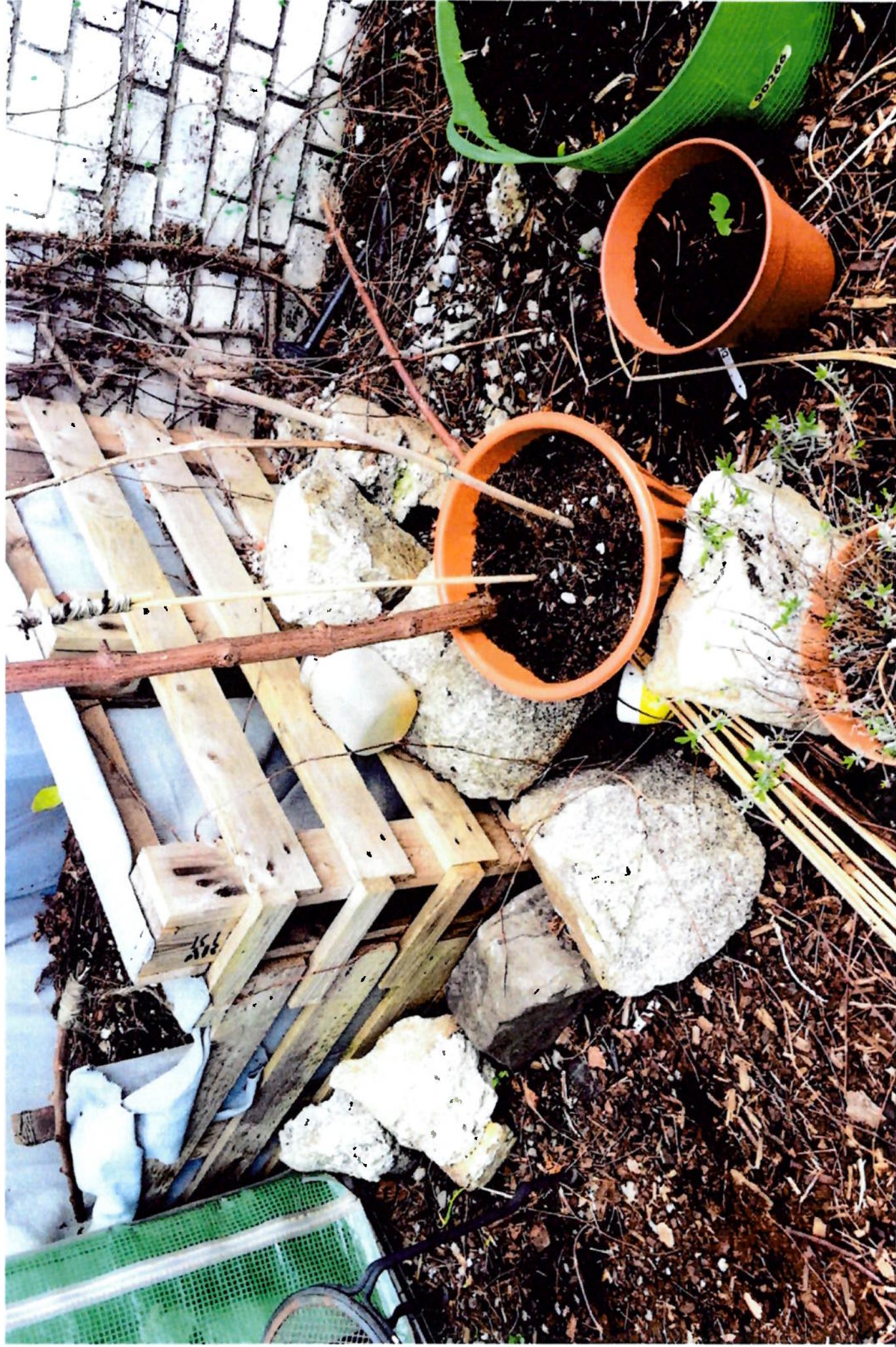
Rubble from wall to Railway Line falling into garden of 16 BERGBOUGH AVENUE, DUBLIN 3 PHOTO No 2
